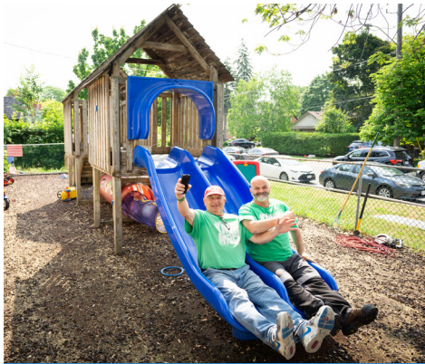
Harvey and Tony take one last slide down the playground structure before we demolish it!
